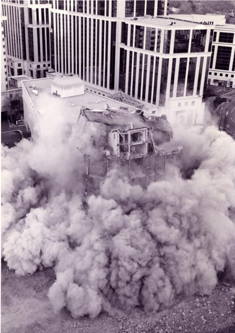
Implosion of County Courthouse, 2/23/97, (Debbie Ernst). Courtesy of the Center for Local History, Arlington Public Library.
